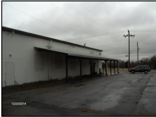
Area of the covered main entrance along the northeast side of the Site building.
