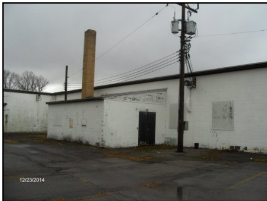
Area of boiler room along the northeast side of the Site building.
