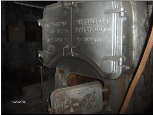
Coal-fired boiler in the boiler room portion of the Site building.
